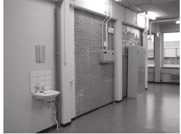
FIGURE 1: Photograph of the corridor wall.
